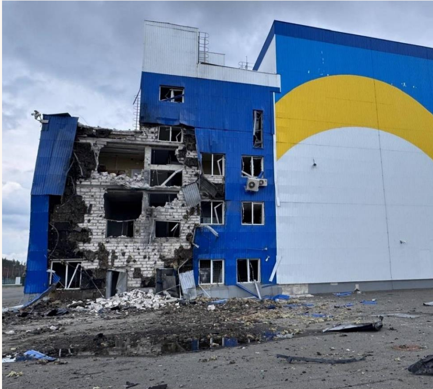
Damaged building of the Centralized Spent Fuel Storage Facility (CSFSF), Chornobyl, June 2026. Photo: Energoatom
